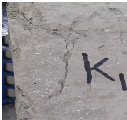
Fig. 12. Cracking in a sample without fibers.
