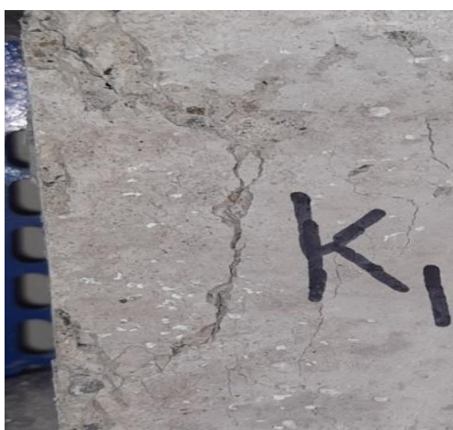
Fig. 12. Cracking in a sample without fibers.
