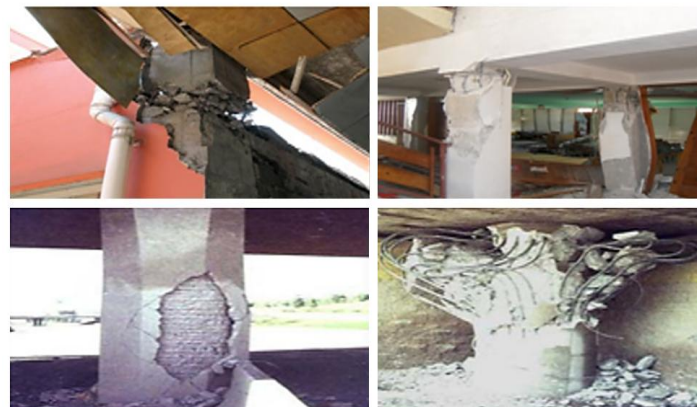
Fig. 2. The failure of the columns.
