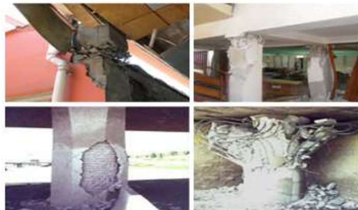
Fig. 2. The failure of the columns.
