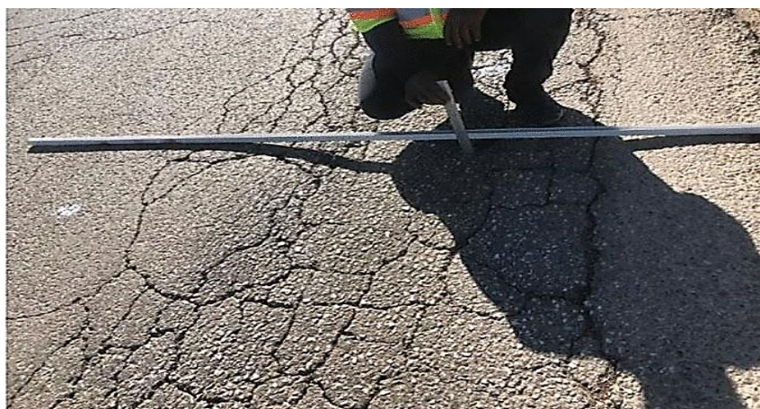
Fig. 7. Road pavement rut detection [59].
