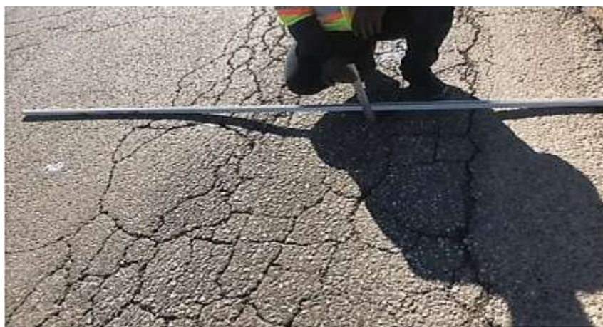
Fig. 7. Road pavement rut detection [59].
